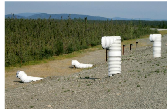
Inlets and outlets of the longitudinal culvert system, Beaver Creek experimental road site (Guy Doré, 2010)
