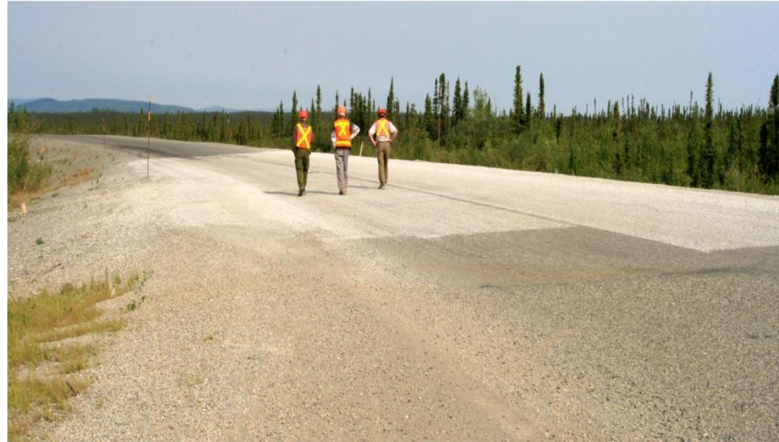
A bituminous surface treatment using light-colored aggregates in the Beaver Creek project (Guy Doré, 2010)
