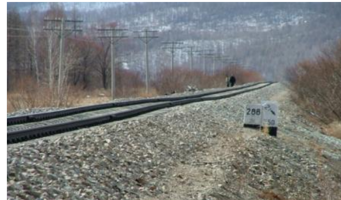
Uneven Thaw settlement in Railway
