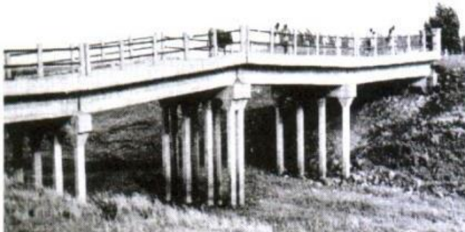
Uneven Frost Heave in Bridges
