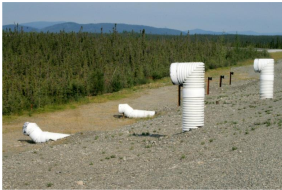
Inlets and outlets of the longitudinal culvert system, Beaver Creek experimental road site (Guy Doré, 2010)
