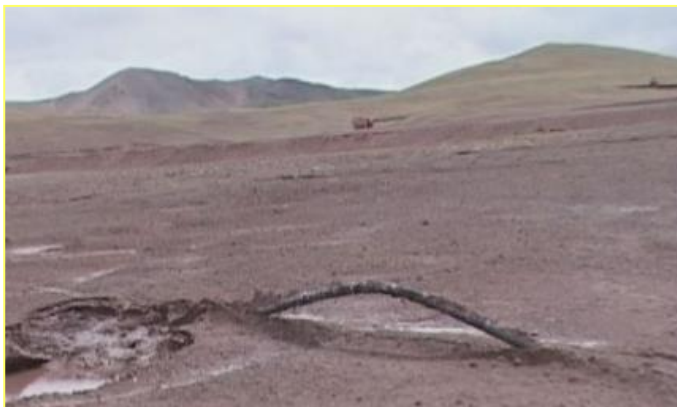
Frost Heave Damage in Oil pipeline
