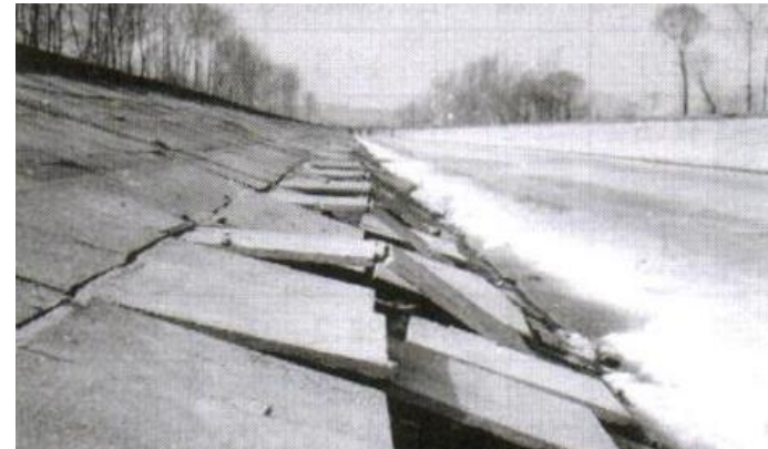
Frost Heave Damage in Channel Lining
