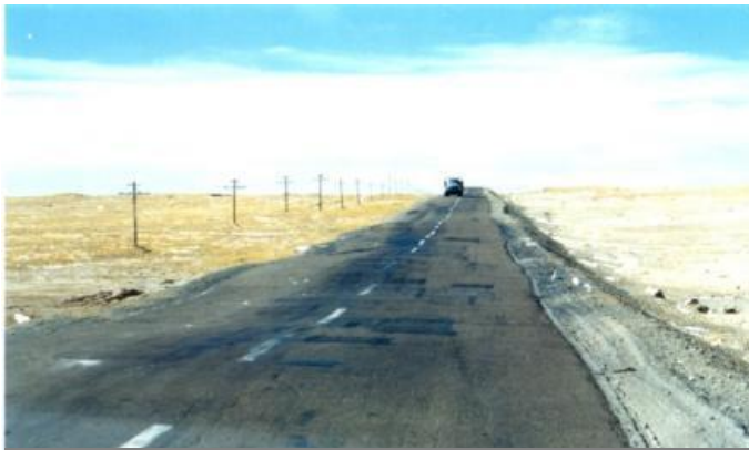
Uneven Thaw settlement in Highway
