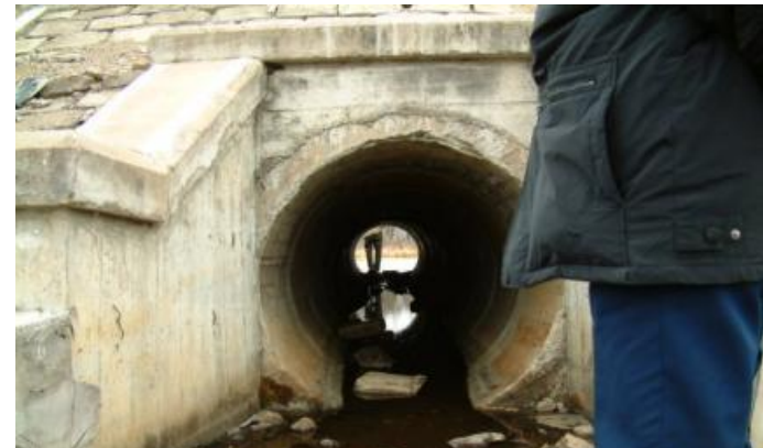
Thaw settlement in Culvert
