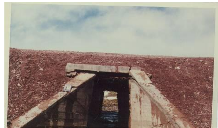
Frost Heave Damage in Culvert
